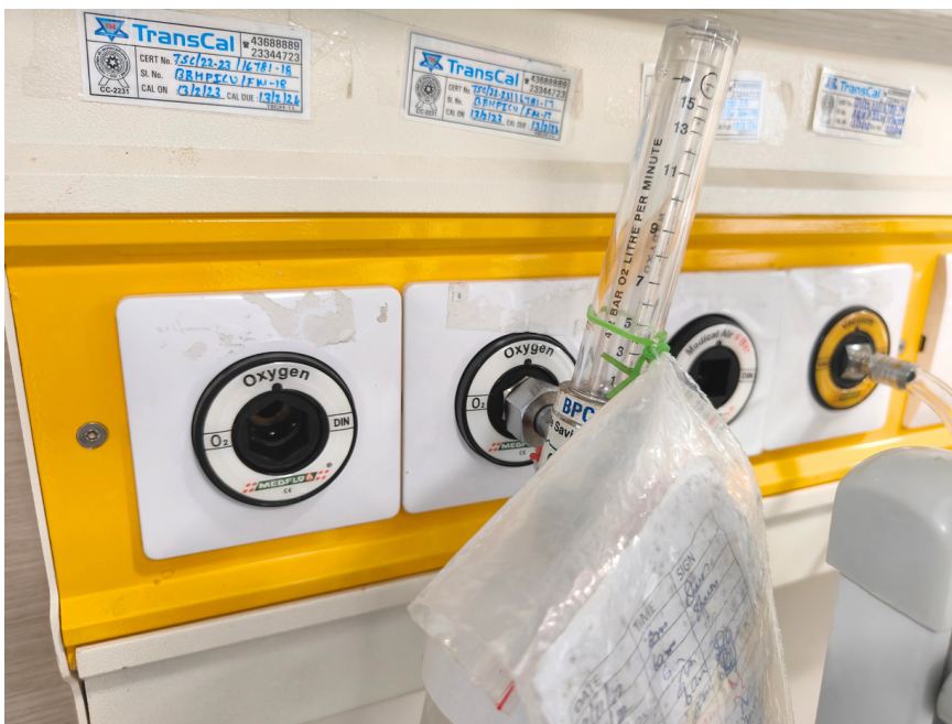
Pipes from which oxygen is supplied to patients
